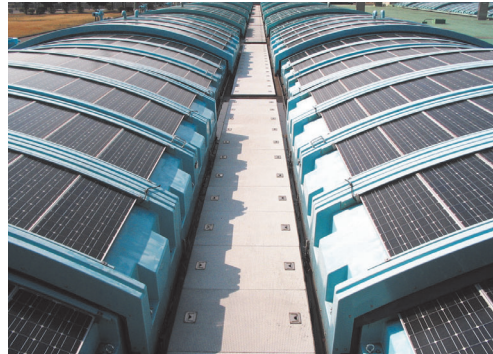
A movable solar power generation system above a filtration basin (Kosuzume Purification Plant)
