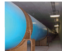
1,350 mm-diameter water pipe inside the utility tunnel
